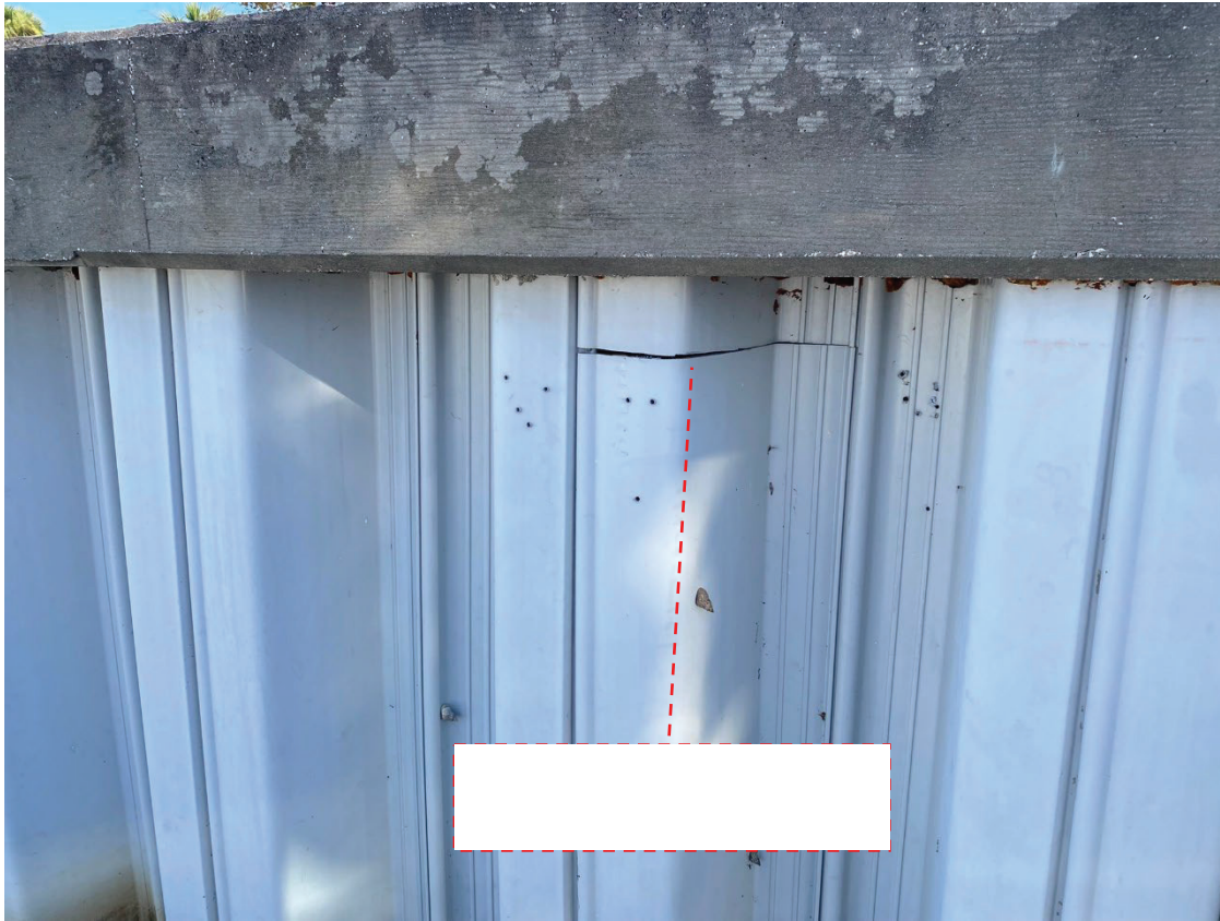
Photo #13 – View of Cut in Vinyl Sheet Pile Below Cap.
