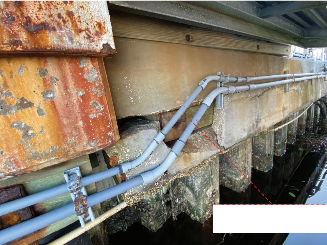
Photo #17 – View of Spalling in Wrap Cap.
